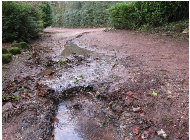
Figure 7 Previous poor state of path network
